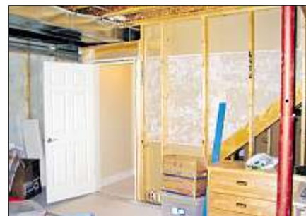
Photo courtesy of CHBA-Calgary Region Renovator of the Year — Albi Renova captures the top honour for a renovator.
