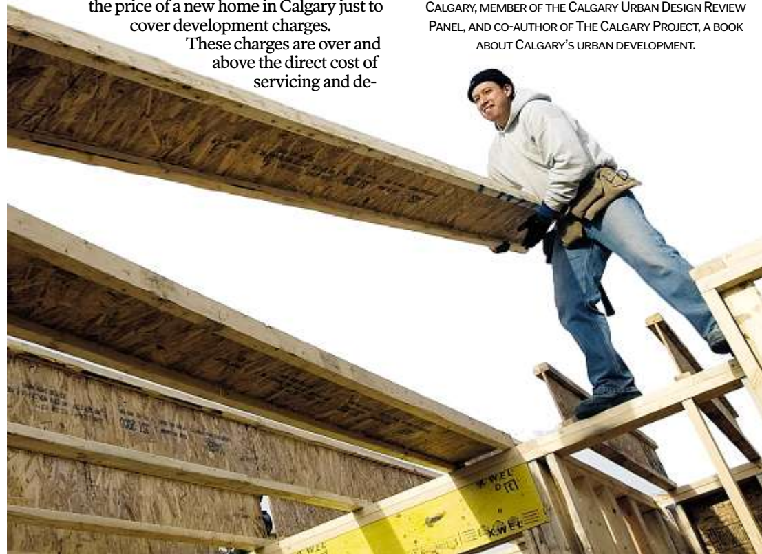
A residential construction worker helps build a house in Elgin Village in southeast Calgary.
