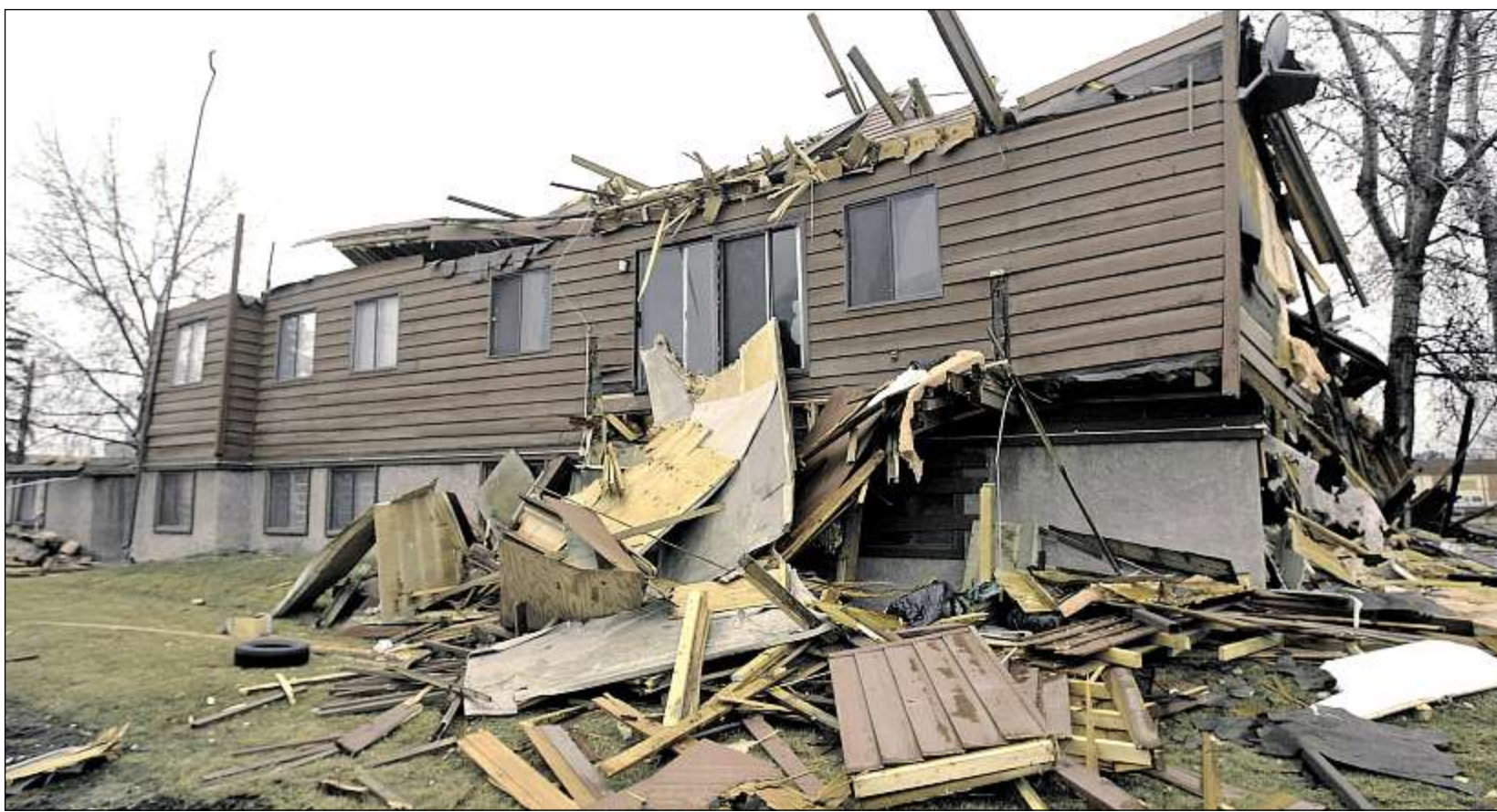
An apartment complex in Victoria Park in the process of being torn down in 2006 as part of the expansion of the Calgary Stampede. Photos, Calgary Herald Archive
